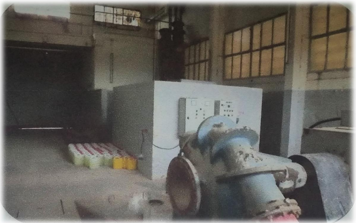
Figure (2.2) : La station de pompage C2.
