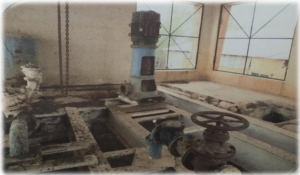
Figure (2.1) : La station de pompage C1.
